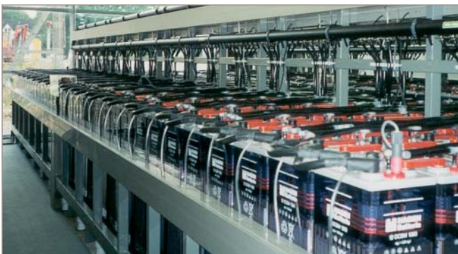
Fig. 7. A 1 MW, 1.2 MWh lead–acid battery installation at Stadtwerke Herne in Germany
