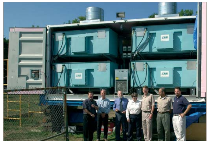
Fig. 11. A 400 kWh ZBB mobile zinc–bromine battery at Lum, Michigan (source: ZBB)
