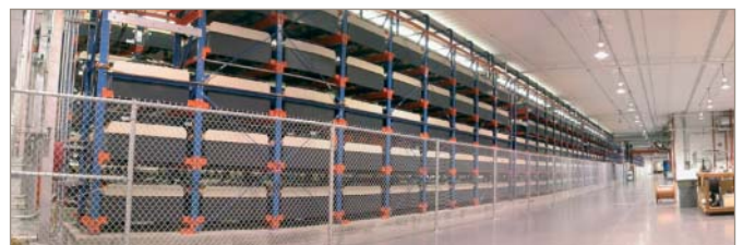
Fig. 8. This Saft 27 MW, 14 MWh nickel–cadmium battery system built in 2003 provides spinning reserve for the Golden Valley Electrical Association in Fairbanks, Alaska (source: Saft)
