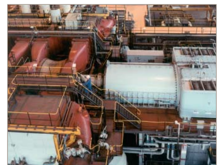
Fig. 2. The 2000 MW Didcot A power station in Oxfordshire, commissioned in 1970, was among the first to use 500 MW generating sets. It has been converted for oil and gas firing as well as coal
